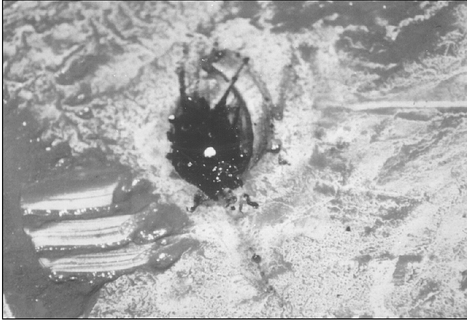
Figure 9-2 Active corrosion penetrated this \frac{1}{4} -in. (6-mm) steel tank bottom in 9 years. Periodic inspections and washouts would have revealed and prevented this problem well in advance of failure
