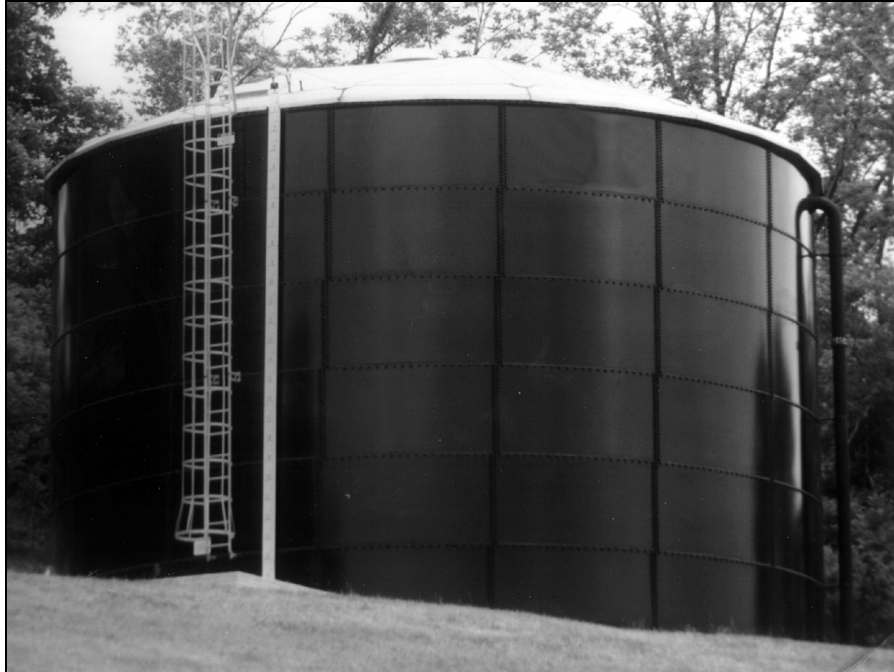
Figure 1-3 Bolted steel reservoir, glass fused to steel
