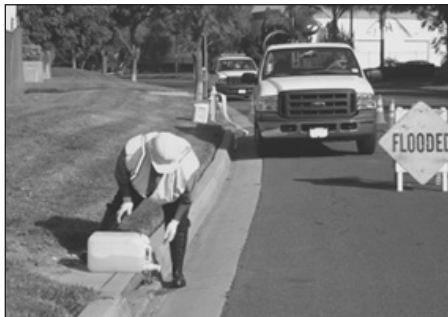
Dechlorination container is placed between hydrant and nearest storm drain. Open valve on container to allow solution to drip out.
