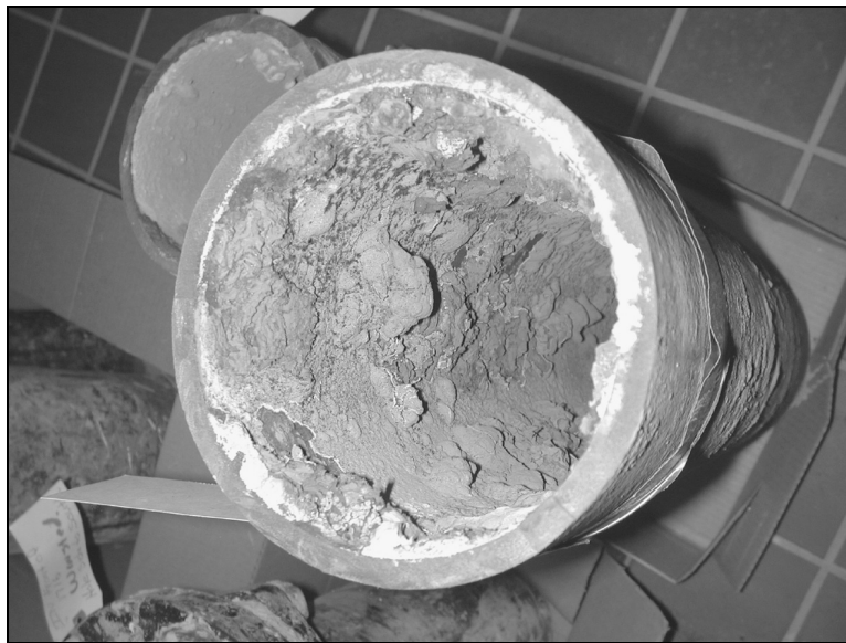
Figure 8-17 Section of distribution pipe where extensive iron corrosion and nitrification were occurring
