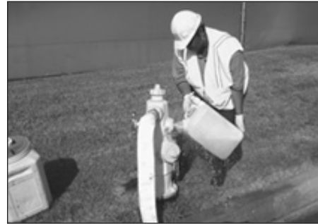
Dry dechlorination chemical is added to the container and then water is added to dissolve the chemical.
