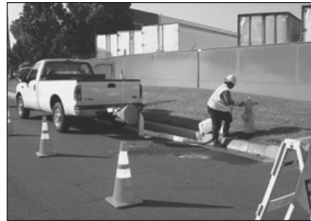
Install the fire hose to the diffuser and then to the fire hydrant.
