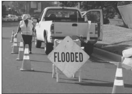
Put on a safety vest and hardhat. Place "Flooded" signs and cones around work area.
